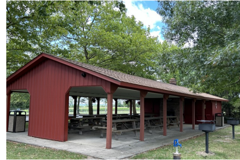
Large Pavilion with new siding, new paint, new grills and new well.
